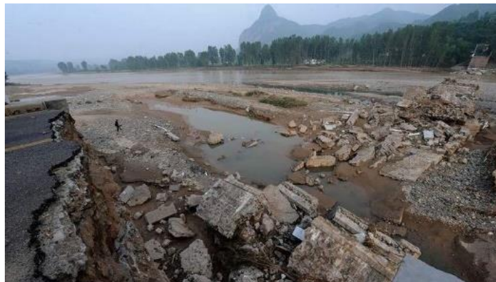
Figure 3. Collapse of Tangying Bridge.
