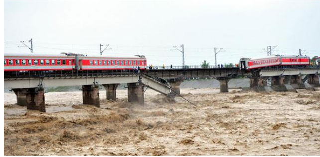
Figure 4. Failure of Shiting River Bridge.
