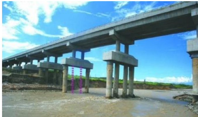
Figure 5. Failure of Mianzu Bridge.
